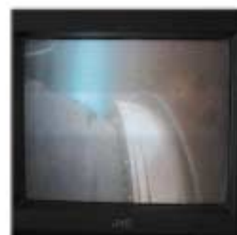
A question of millimetres: Attaching the breakwater into an 8 m diameter steel ball and socket joint 9 m beneath the water level.
